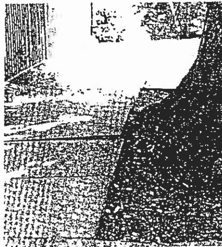
PAVING SLAB TREE DAMAGE
