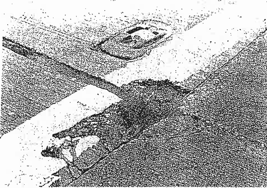
CRACKING, PLUCKING AND LOSS OF MATERIAL IN CONCRETE CARRIAGEWAY
